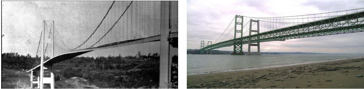
Figure 6: The collapsed Tacoma Bridge and the current twins Tacoma Bridges.
